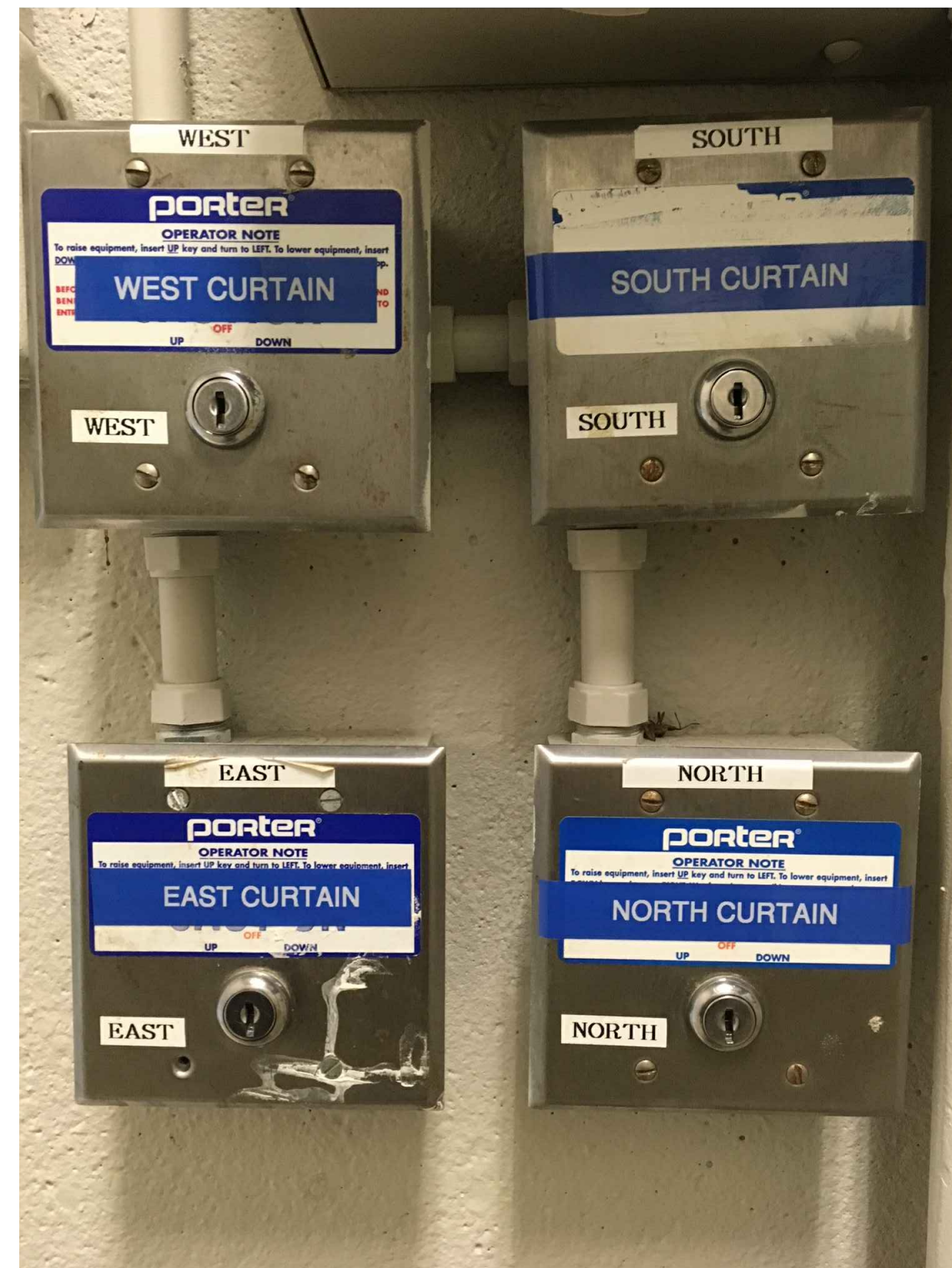
EXISTING CURTAIN CONTROL BOXES
